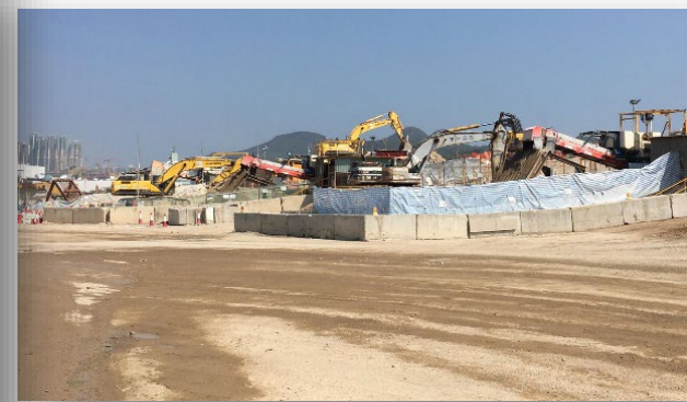
破碎混凝土及石塊可循環再造成200級再造石填料 Recycling of broken concrete and rock pieces into Grade 200 recycled rockfills
